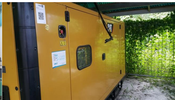
Gambar 5. 36 Genset Baru RSU Sofifi
